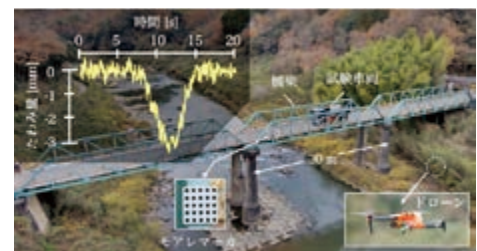
橋梁のたわみ計測の検証実験 Verification experiment of bridge deflection measurement
