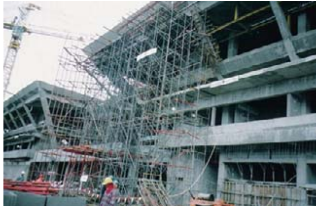
Fig. 16: Second laboratory building. Construction of the overhang to prevent strong sunlight was quite a difficult work.
