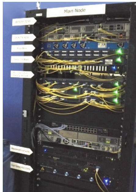
Fig. 2(b): Exterior view of the standard rack with some of blades (hereinafter referred to as the “standard blade”)
