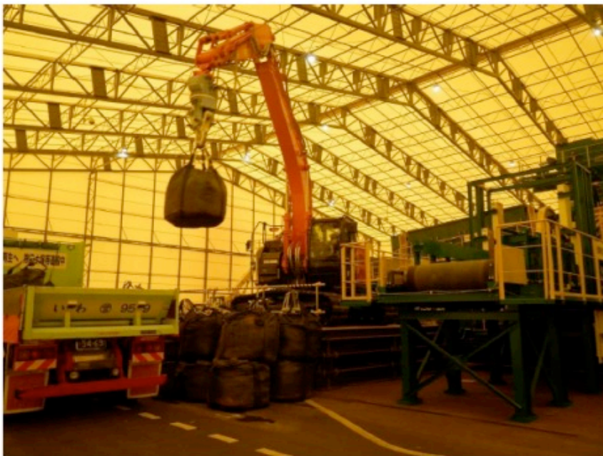
Reception/Separation Facility (First period in Futaba) (Processing capacity 140t/h)
